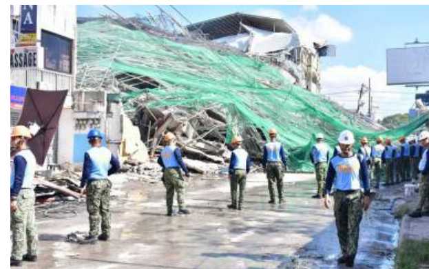
COLLAPSED. Philippine National Police (PNP) personnel secure the site of a collapsed nine-story building in Angeles City, Pampanga, in this undated photo. The Department of Social Welfare and Development on Saturday (May 30, 2026) warned the public against scammers claiming to be beneficiaries of DSWD assistance. (Photo courtesy by PNP)
