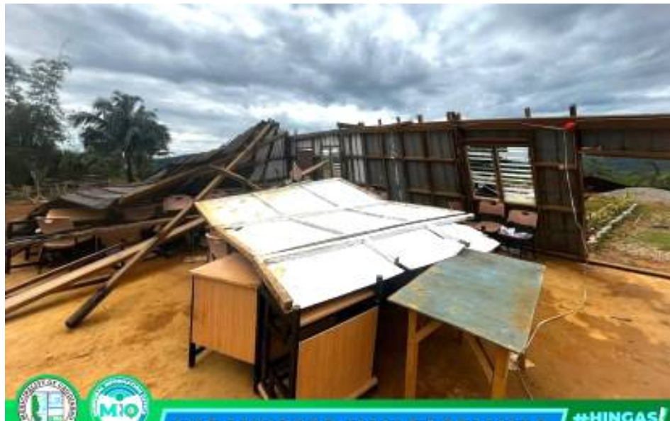
PREPARATION AND RECOVERY. Barangay Sta. Rita National High School in Cagadiano, Dinagat Islands suffered severe damage following the onslaught of Typhoon Tino (international name: Kalmaegi) on Tuesday. The Department of Education on Friday (Nov. 7, 2025) assured that it is preparing for the possible impact of Uwan while continuing recovery efforts in public schools affected by Typhoon Tino. (Photo courtesy of Facebook/ MIO Lungsod Nan Cagadiano)
