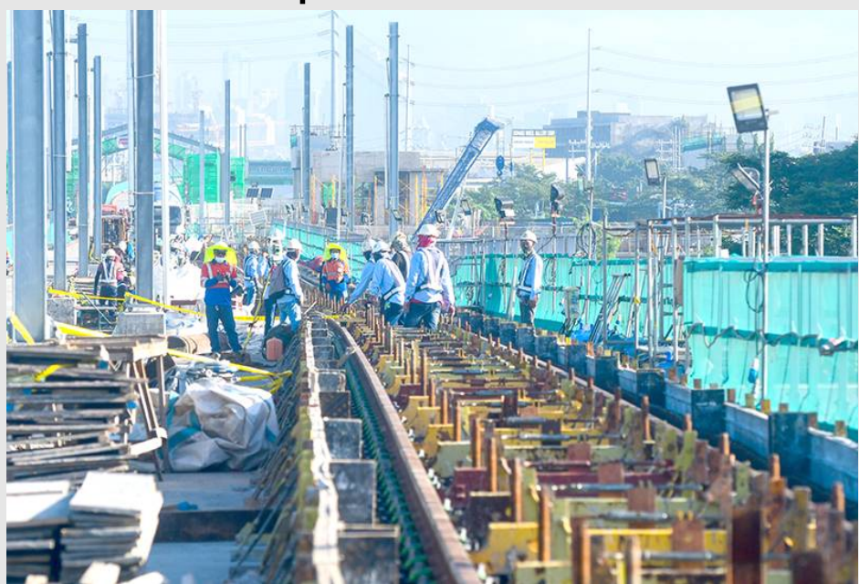
Department of Transportation, Light Rail Transit Authority (LRTA) and Light Rail Manila Corporation (LRMC) officials inspect the ongoing work at the LRT-1 Cavite Extension Phase 1 in Parañaque on November 14, 2022. The extension project is targeted to be finished by 2024. Mark Demayo, ABS-CBN News
